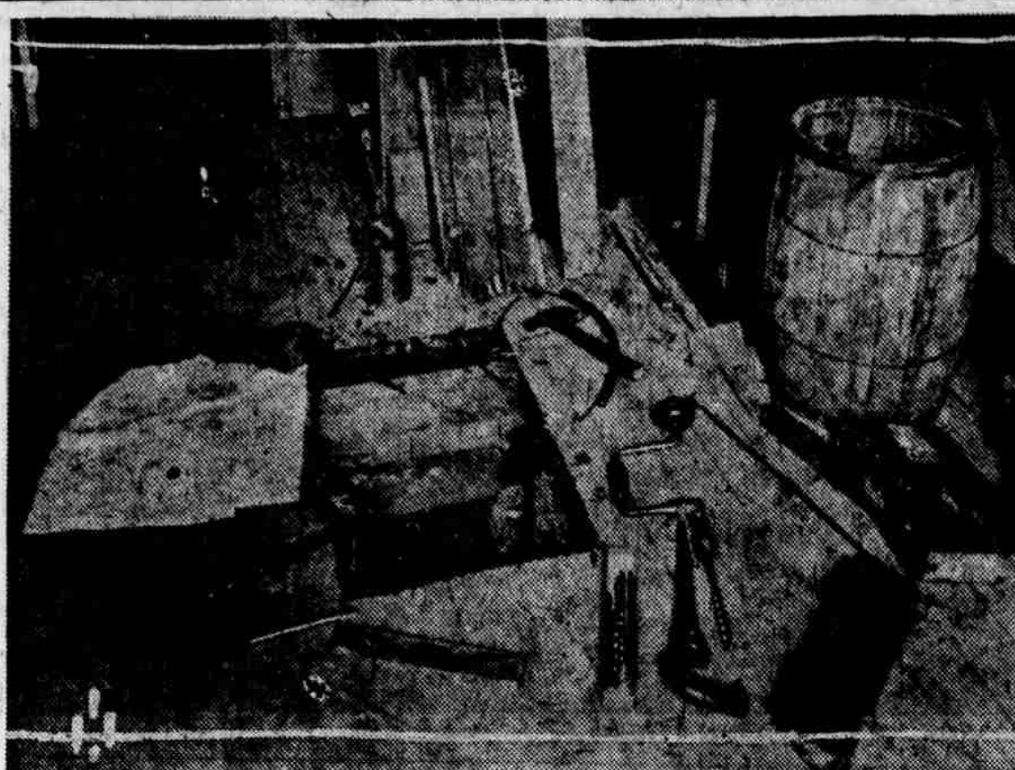
This shows the hole bored through the steel ceiling of the Morris Deiches Sample Cloak and Suit company, 216 North Sixteenth street, early yesterday morning by burglars, who escaped with $2,500 loot, which has been recovered. The tools lying around were taken from the studio of the Ernest Bihler photograph concern, through whose transom the burglars entered. Photograph by Bihler.
