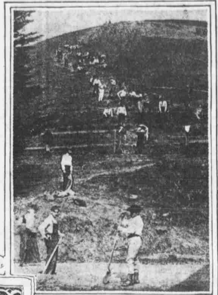
"Charter Day" Carrying rock and cement up Charter Hill to build the big 'C'.
