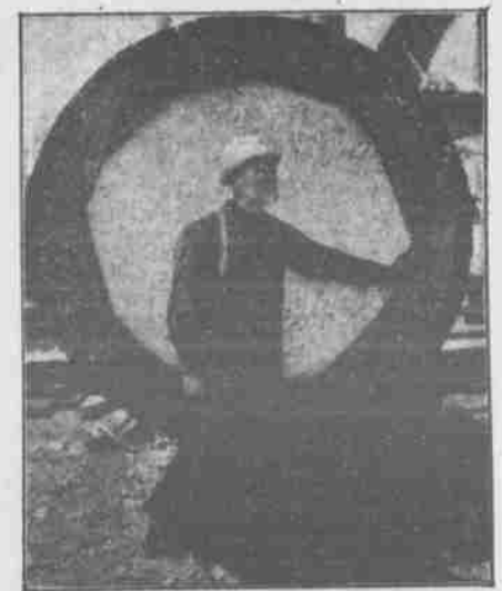
W. F. HOWLAND, THE VETERAN STONE SETTER, STANDING BY THE BASE OF ONE OF THE BIG COLUMNS.
