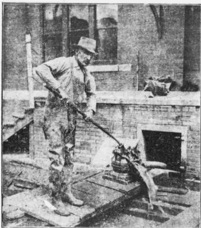
PUMPING OUT THE "BILGE WATER" FROM A WHOLESALE GROCERY ON BROADWAY.
