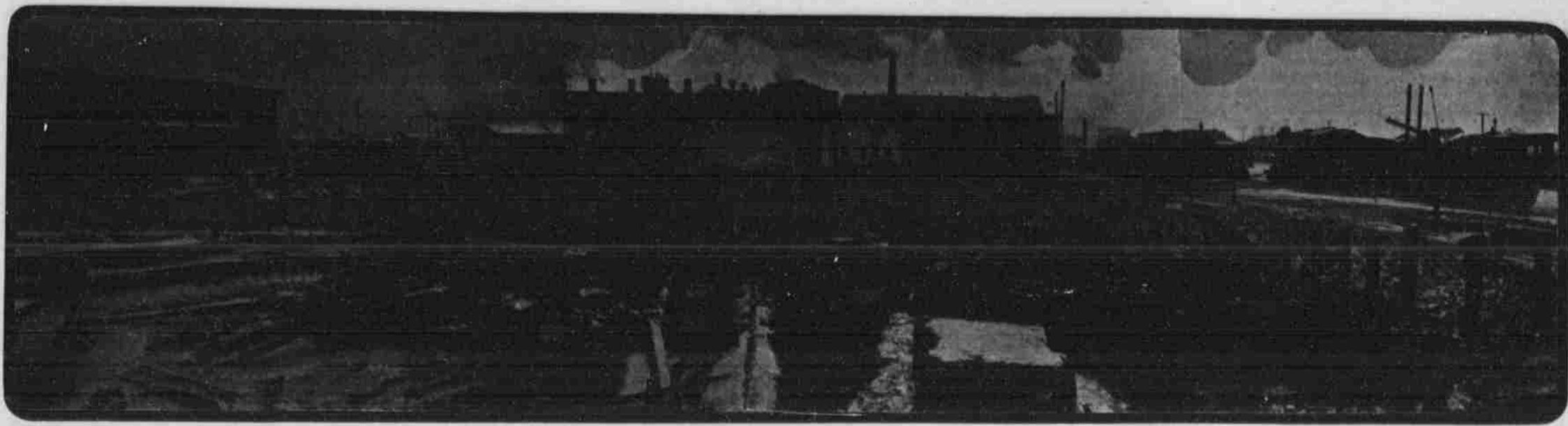
GENERAL VIEW OF THE UNION PACIFIC SHOP YARDS IN OMAHA, WHERE THE GROUND IS BEING CLEARED FOR THE ERECTION OF A MACHINE SHOP TO COST THREE-QUARTERS OF A MILLION—Photo by a Staff Artist.
