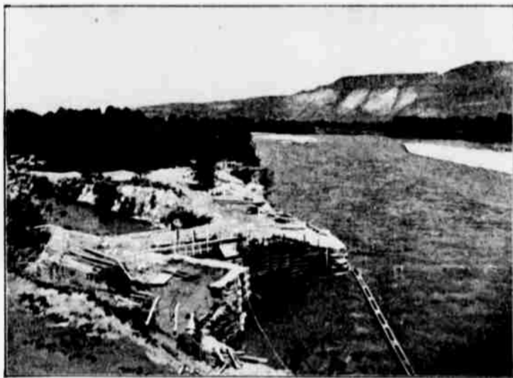
Live Stream Irrigation System on Union Pacific in Nebraska.
