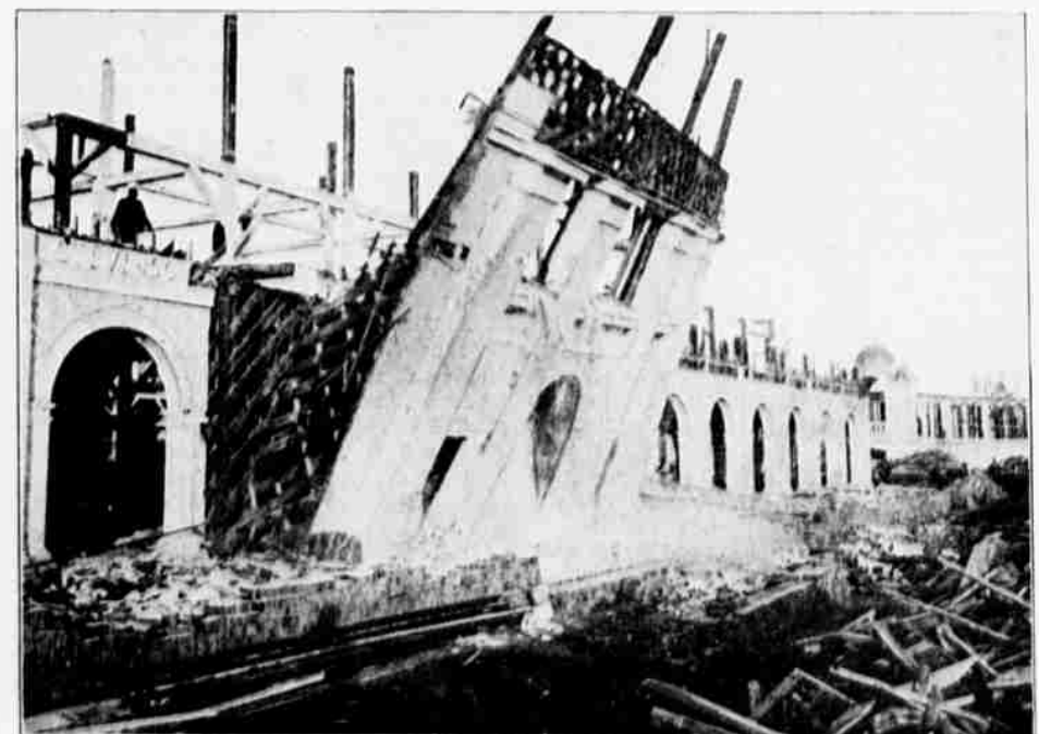
WRECKING THE EXPOSITION—FALLING OF SOUTH ENTRANCE OF MACHINERY HALL—Photo by Louis R. Bostwick.
