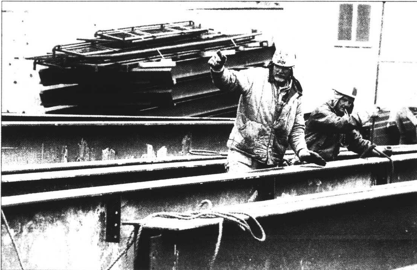
ROY BLEICH, left, and Jerry Bailey, of Davis Erection Company, help a crane operator move steel beams at Memorial Stadium Monday. Construction workers said the day had been going a little slower than usual because of Monday's precipitation. JAY CALDERON/DN
