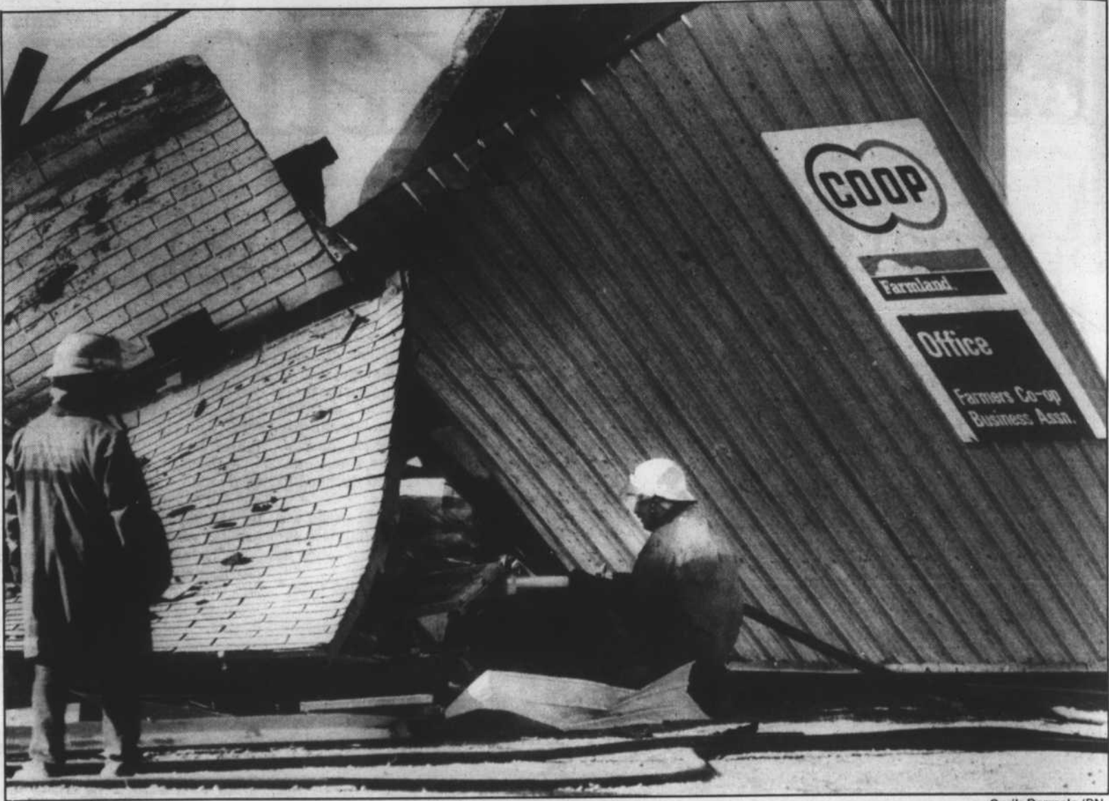
Fire fighters work to extinguish a hot spots after an explosion ripped through a grain elevator office early Tuesday afternoon in Gresham Nebraska. The explosion injured two people and completely destroyed the office.
