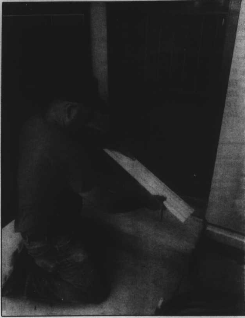
Kenneth Moore of Builders Inc. works on a fire exit from the Coliseum swimming pool.
