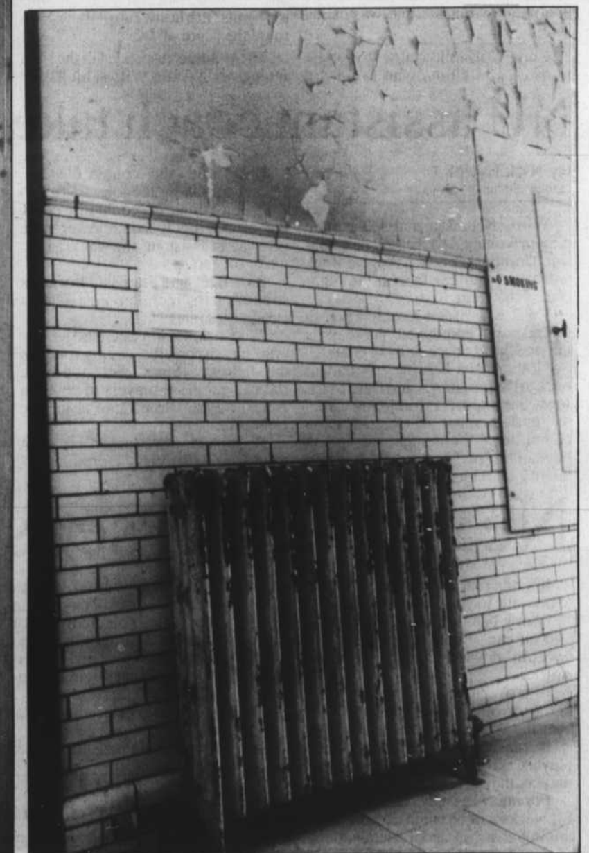
The most noticeable flaw in Richards Hall is the constant high temperature, students say. The heaters are always on, winter or summer. Students say the building is always hot even in the winter.
