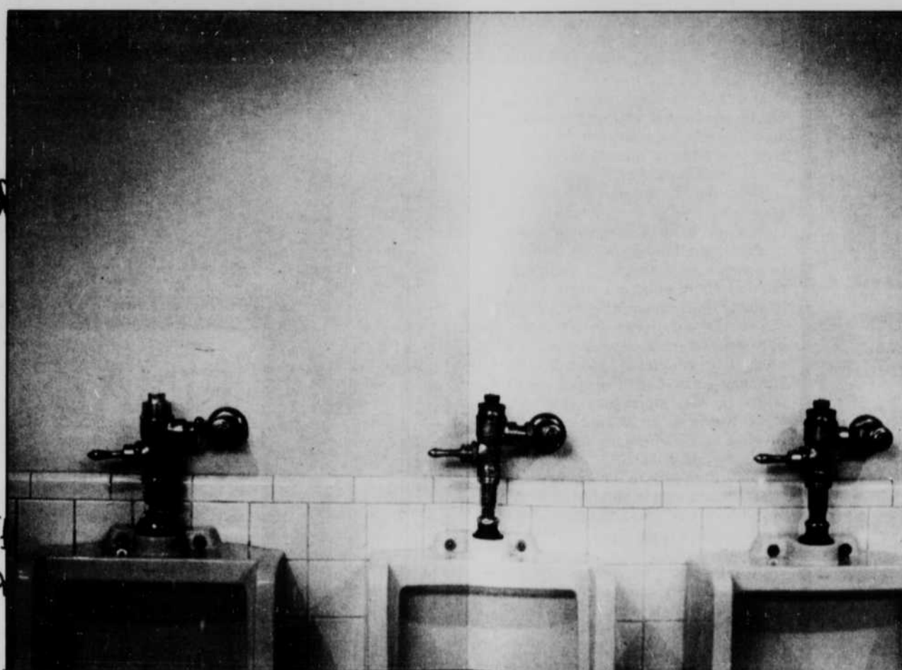
The bare walls of Ferguson's men's restroom. Butch Ireland/Daily Nebraskan
