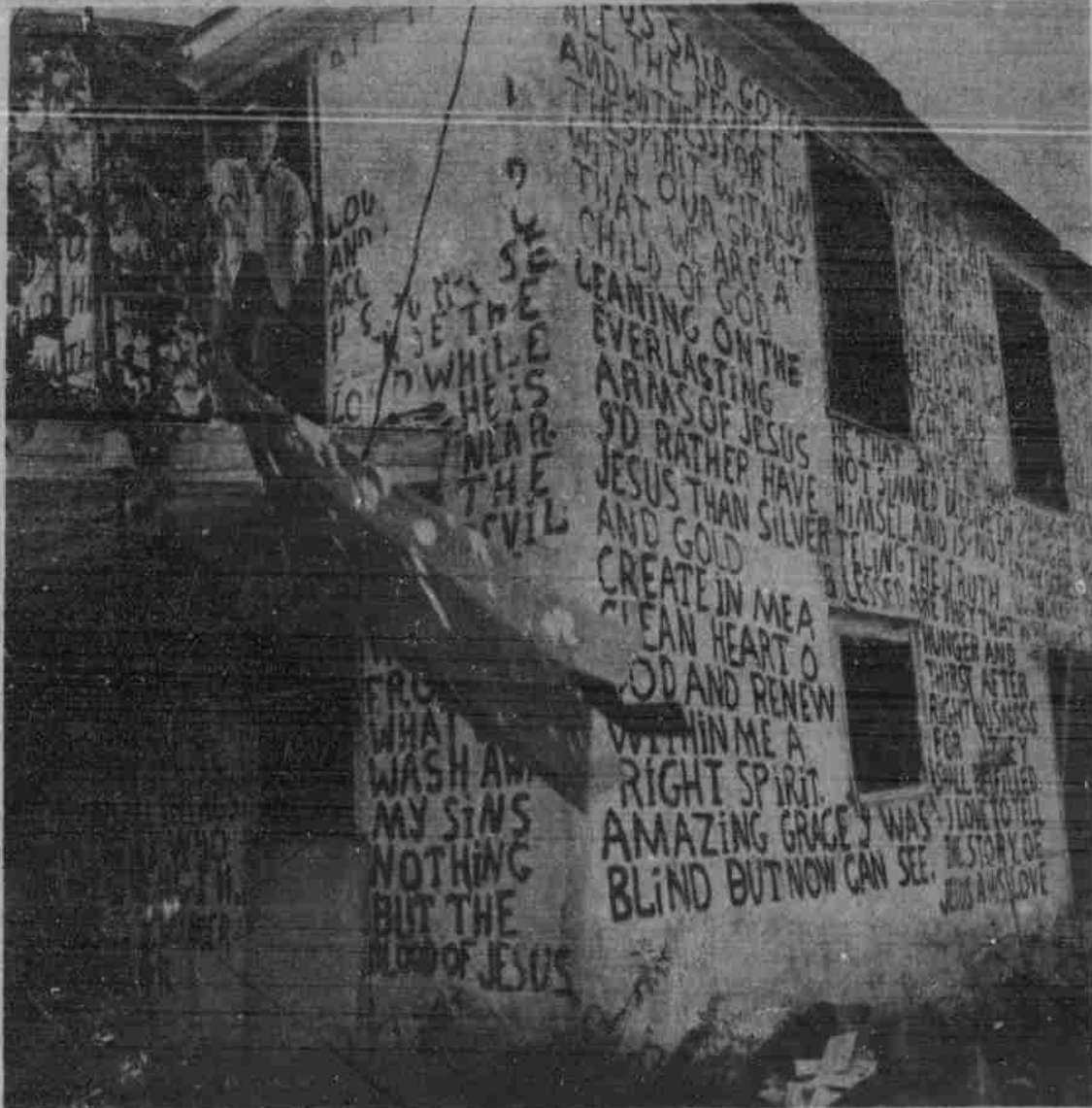
Volunteers helped clean up the condemned Martin Lindell home last weekend.
