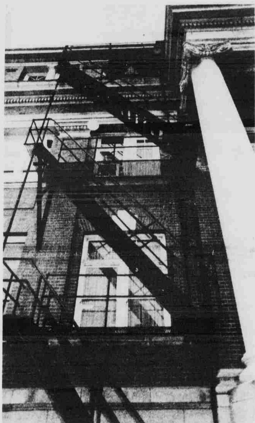
The Temple Bldg. contains some of 48 remaining UNL fire hazards.
