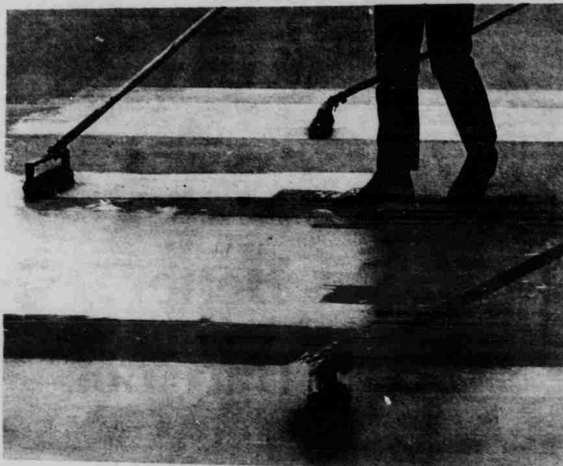
More tennis courts on the way . . . workmen surface the new tennis courts south of Harper-Schramm-Smith dormitory complex.
