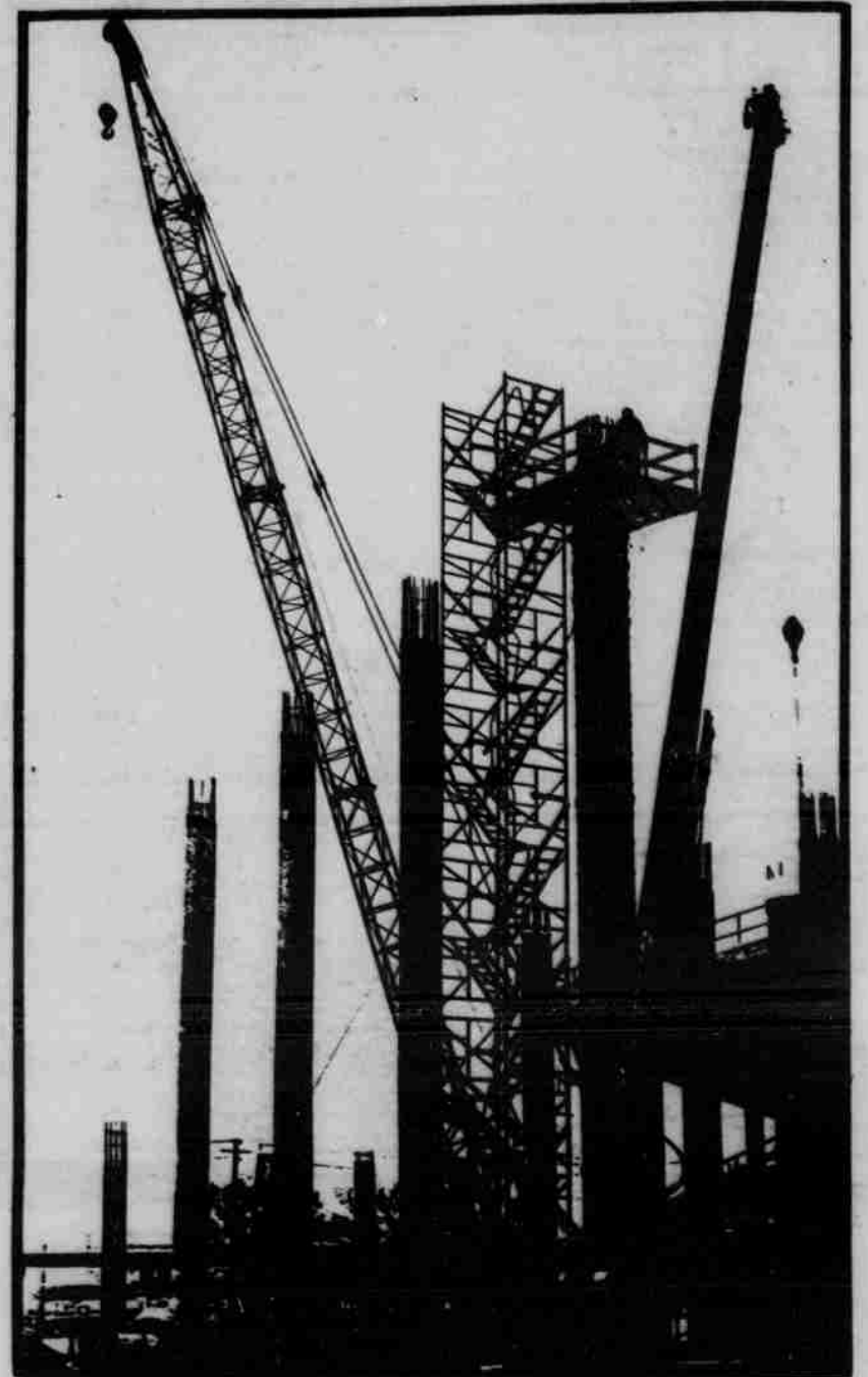
More Big Red seats... construction is proceeding rapidly on the addition of 9,400 seats to the south end zone of Memorial Stadium.
