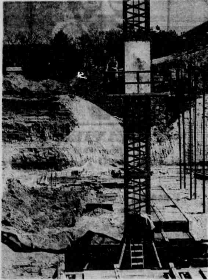
Barricades are near completion as East campus "digs-in" to preserve their vital bodily fluids. Workmen here complete a span as loud cheers ring from both sides.
