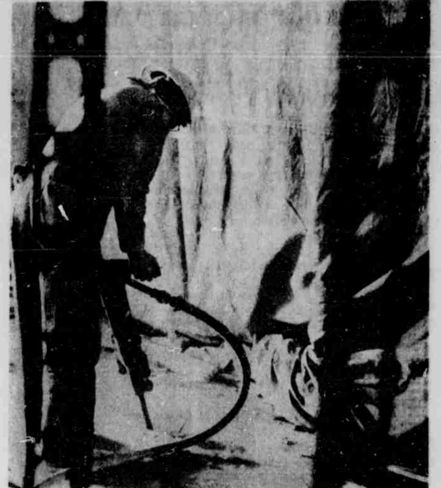
Construction is underway on the new undergraduate library to be located on the first floor of Nebraska Hall. Completion date is set for September, 1969.
