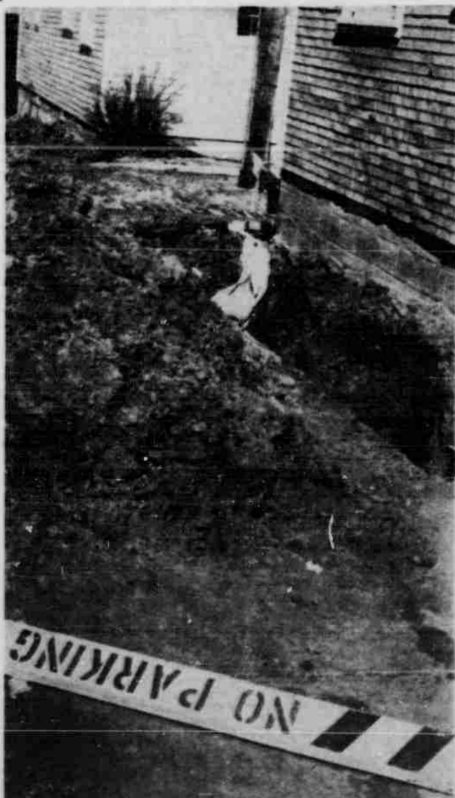
LAYING ELECTRICAL CABLES . . . causes consternation underfoot as students must avoid the holes in the sidewalks.
