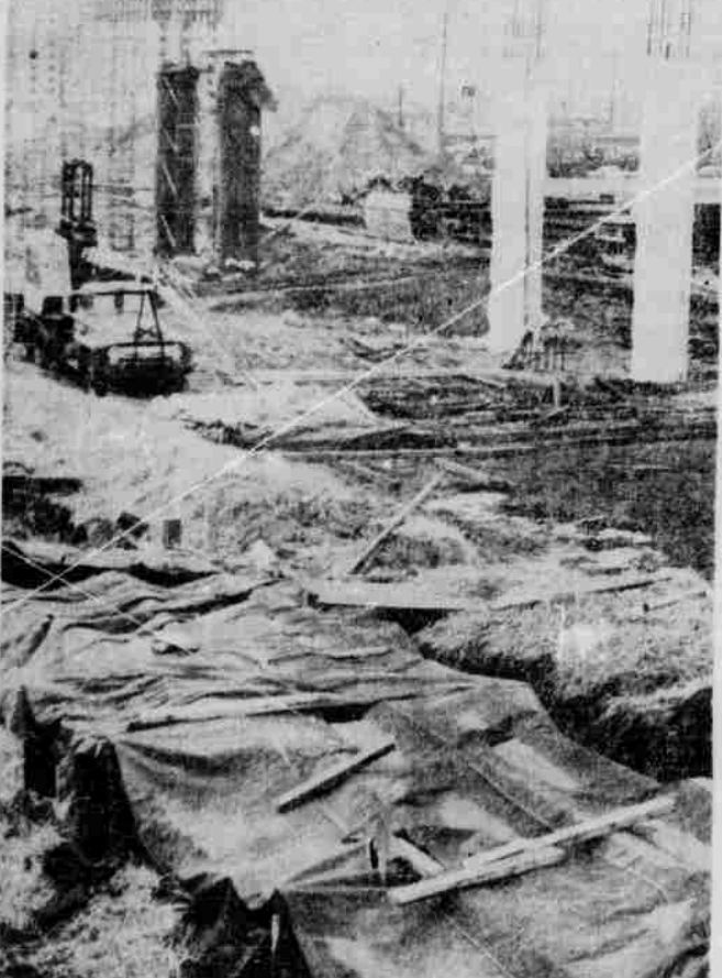
CONSTRUCTION UNDERWAY . . . on the women's new physical education building which is expected to boost women's sports participation.
