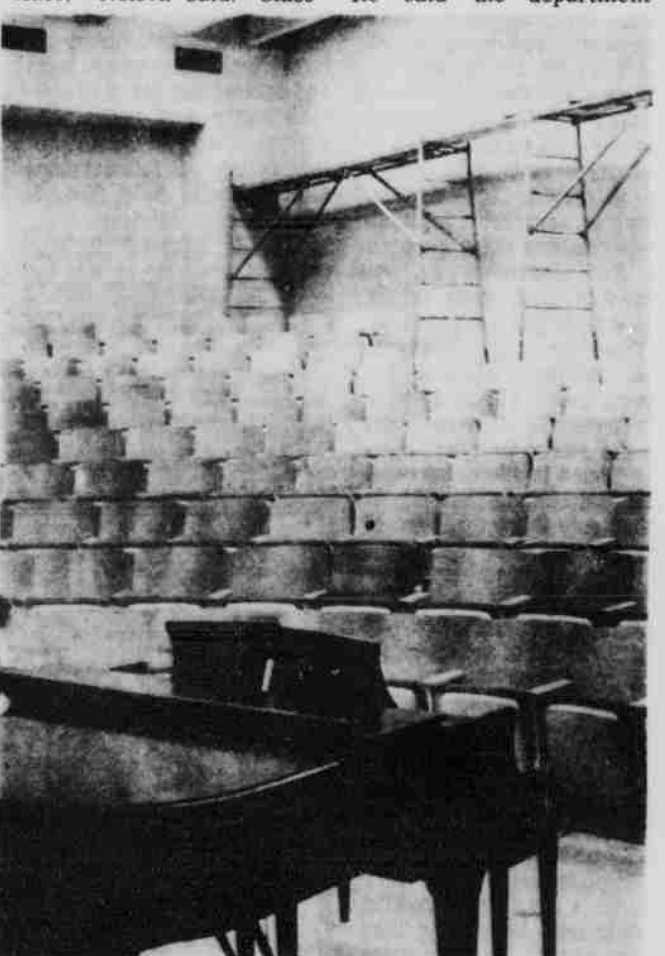
While work continues in empty rooms as the Music Building nears completion.
