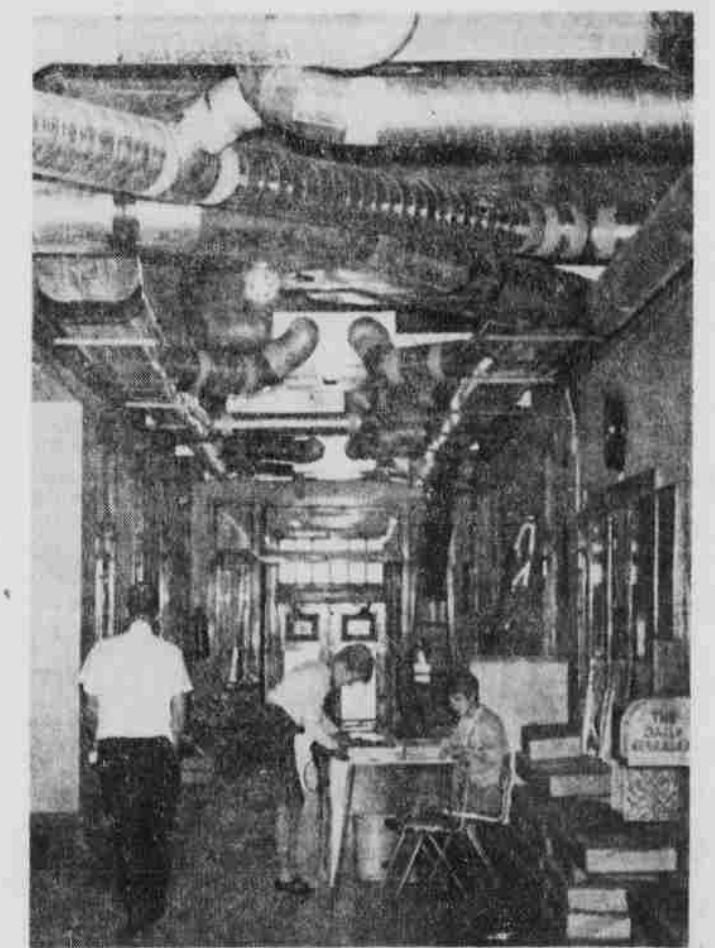
EXPOSED PIPES . . . in Teachers College indicate installation of new air conditioning and heating system.
