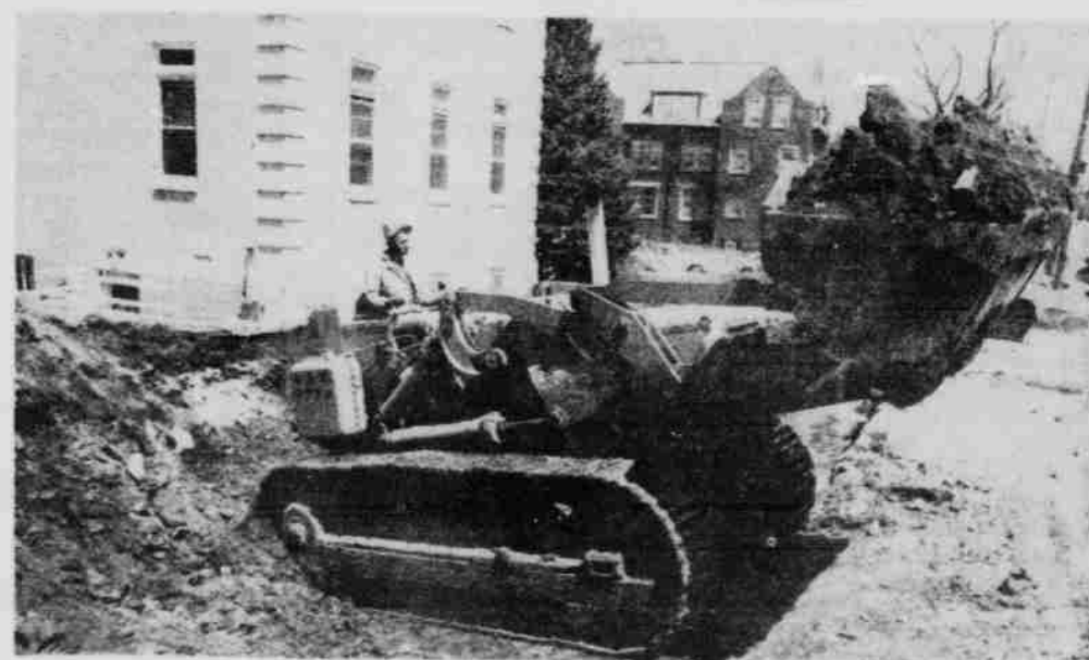
WORK HAS BEGUN... on a three-story addition to the Phi Delta Theta fraternity house. The new wing will include a kitchen, dining room bedrooms and a sundeck.
