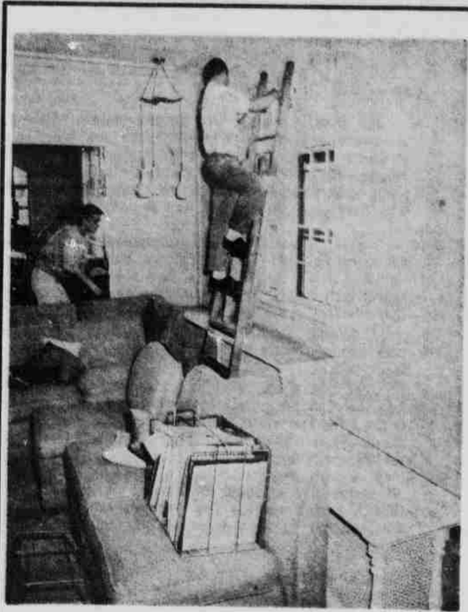
REPAIRMEN . . . are at work this week repainting the living room of the Tri-Delt sorority house following a fire in the house last Monday. The kitchen and basement suffered heavy smoke damage. The sorority members moved back into the house last Saturday. No estimation of fire damage has been made.
