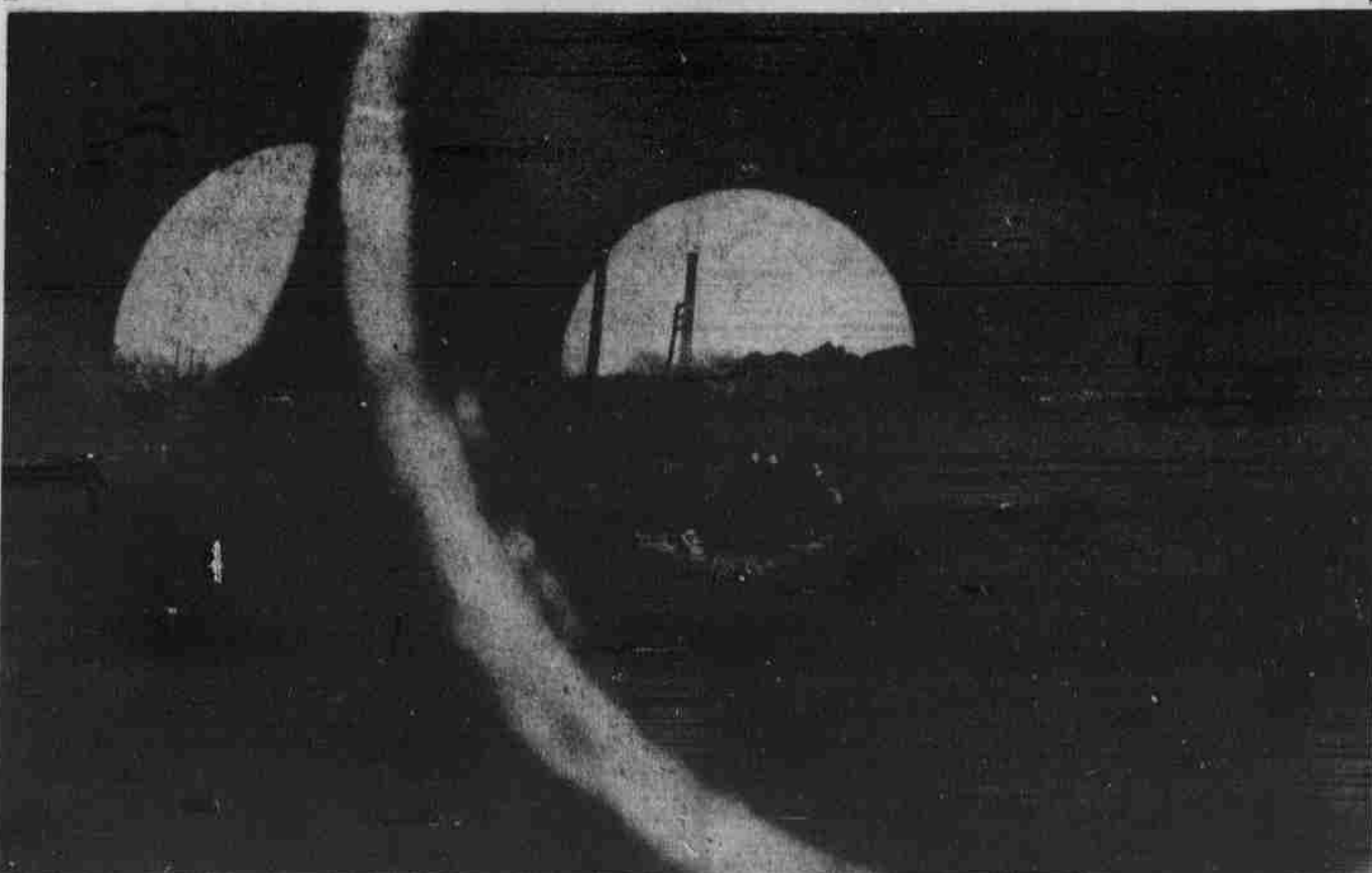
CONSTRUCTION SEEN THROUGH A PIPE — A glimpse of the construction activity at the site of the new men's dormitory on 17th street can be seen through a section of pipe for the new building's sewer system. The pile of earth in the background is from the excavations for the basement and foundations. The picture was taken by Sue Leonard for a Journalism Photography class.
