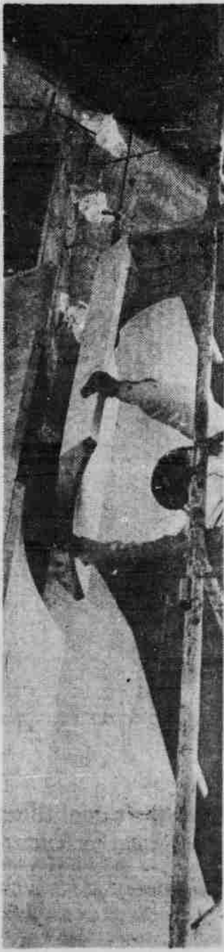
Photos by Doug McCartney MARBLE SLABS for facing on the new Sheldon Art Gallery have arrived from Italy and are now being put on the walls. Work is expected to be completed on the Art Gallery in 1963.
