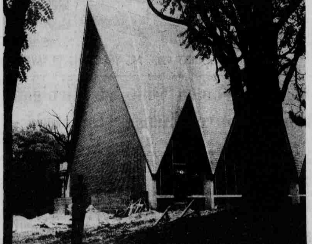
SOMBER SIGHT Many students, as the one pictured, are impressed by the sight of the nearly completed Wesley Center on North 16th Street. Work on the new Wesley Center is nearing completion according to Rev. William Gould. Rev. Gould said there were hopes that they could move into the building before Christmas although the consecration of the new structure will not be held until Feb. 11. The building contains three levels. The lower level houses the kitchen and dining room with the capacity to serve 300 people. The other two levels include four offices, a music room, library, office work room, chapel, a balcony choir loft and special choir room and auditorium, featuring a portable stage, with capacity of 300 people. The chapel features a free standing alter in the shape of a triangle and the student center is roofed by an unusually designed broken cement roof.
