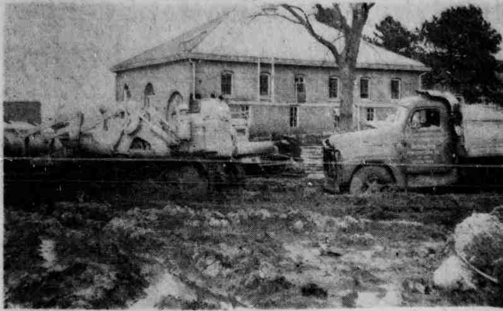
KELLOGG BOGS DOWN—First snow, now mud hampers the workers on the Kellogg Center. Here a husky bulldozer bogs down trying to pull a truck out of the knee-deep quagmire.
