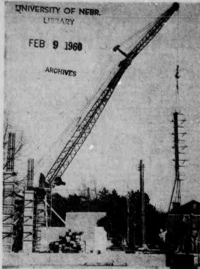
KELLOGG CENTER —Construction got a boost Monday as workmen had spring-like temperatures to their favor. The warm weather is expected to continue for several days. The center is being built on Ag Campus at 33rd and Holdrege.
