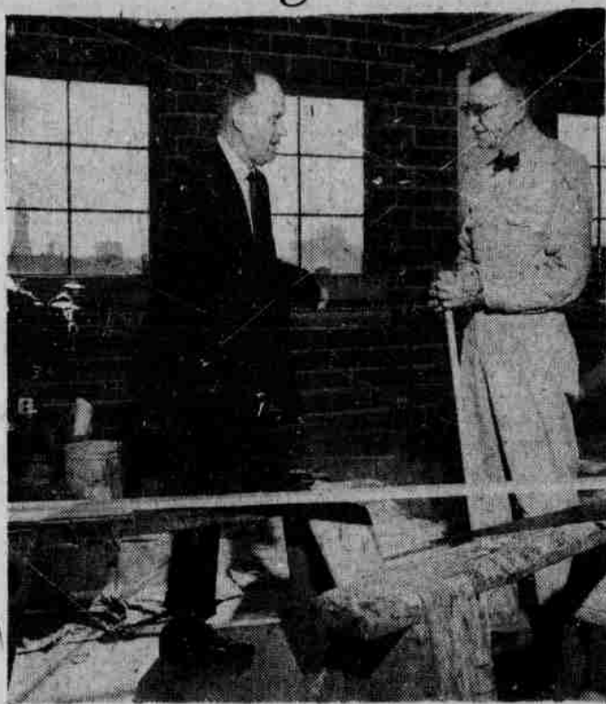
WEATHER BUREAU—Richard Myers (left), meteorologist in charge of the Lincoln Weather Bureau, keeps in touch with O. C. Hirsch, contractor who is putting the finishing touches on the new Bureau quarters in the former Elgin Building. After an absence of four years from the University campus, the weathermen will move back after Jan. 1. The quarters will be in the fifth floor of Elgin, next to the roof.
