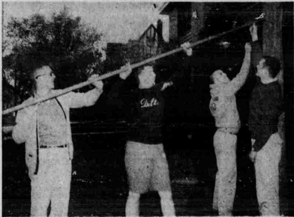
WHATEVER IT IS, it looks substantial. That's what might be said of Delta Tau Delta's homecoming display building at 715 No. 16th St. Steel rods are being attached to a telephone pole by Roger Khrounek (left), Dick McBride, Mick Tooley and Joe McWilliams.
