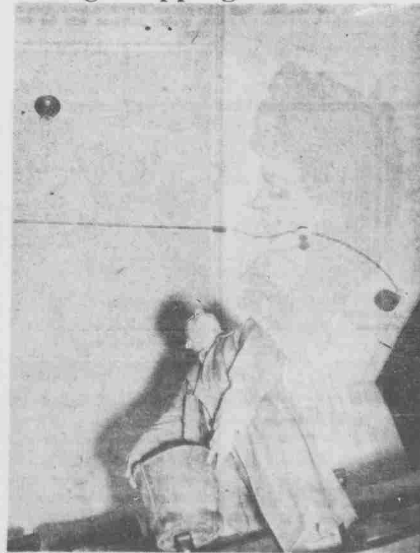
GAYLORD MAER adjusts a bucket to catch the rain leaking through one of many cracks in the auditorium ceiling. The second oldest university theater in the country, the Temple was built in 1904. Watch falling plaster, Gay!
