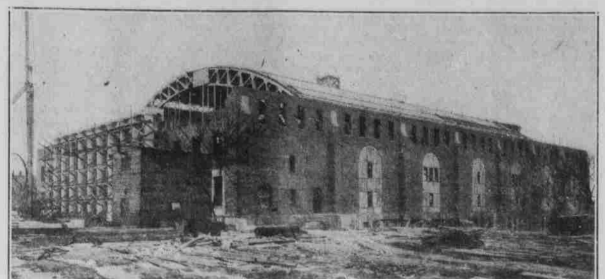
Nebraska's new Field House as it looks at the present time. The structure is practically enclosed and with the heating system installed can be used as soon as the front and rear walls are completed. As the picture shows, the columns and brick wall in front are not yet finished. When completed the building will become the home of Husker indoor sports and University functions.
