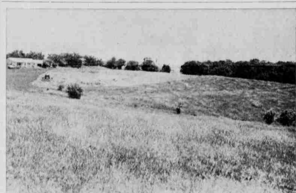
PARK WORK UNDERWAY —Grading and bulldozing at the city's new park site in southwest Plattsmouth has been started. Above a view looking northeast from a point near the water tower shows a dozer pushing earth in the area which has been designated for tennis courts and swimming pool as possible future developments. Earth will be graded from the north and west to fill in the open valley and provide more level ground.
