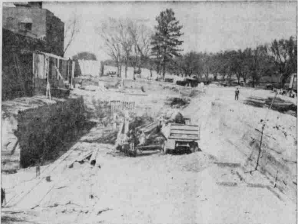
FOOTINGS READIED —Footings were poured this week for the new service wing to be built at the Nebraska State Masonic Home here. The new wing will cost about $330,000 and will give the Home facilities needed now as well as potential for future needs when the Home is enlarged further. According to Superintendent Raymond Evers, the new wing will have com-
