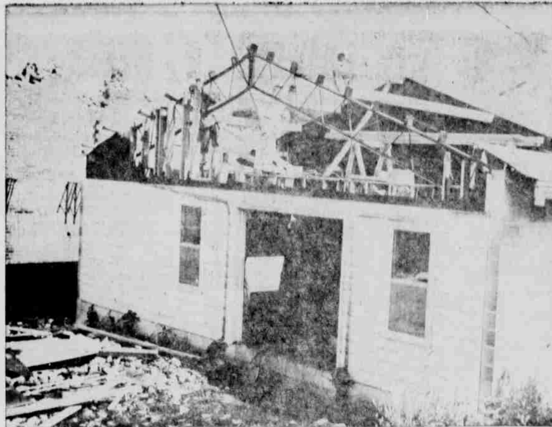
MUSEUM BEING REPAIRED —Work was begun the past week on repair of the Cass County Historical Society Museum here. The north end of the new building was badly damaged by fire June 23 when the Hotel and Theater buildings were destroyed. Young and Jose, contractors who constructed the building, are doing the restoration. Harold Austin of Austin Plumbing and Heating said the cold air return ducts beneath the building's concrete floor had filled with mud and strips of the floor would have to be torn up to clean them out. Some small boys offered to crawl into the ducts Friday to inspect but didn't get far before they encountered mud.
