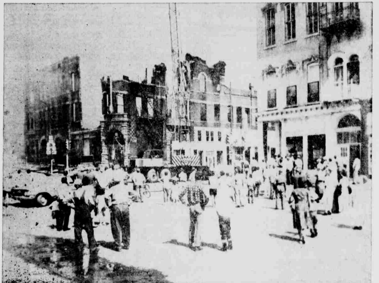
WALLS COME DOWN—Demolition of the Hotel walls for a steel ball was being gently swung from the crane to topple small sections at a time.
