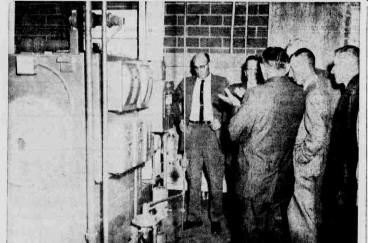
OPERATION OF THE DIGESTER was explained by Cappell (back turned) to from left, Wayne Rodehorst. The men were in the control building. Unit at left is gas-fired furnace used to heat sludge in digester to about 90 degrees.
