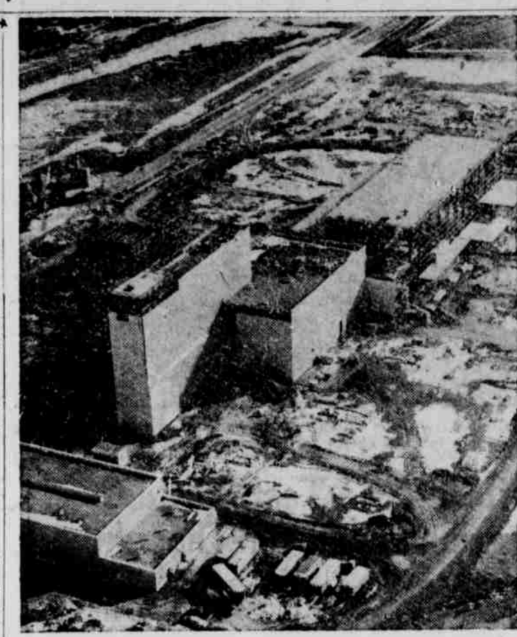
CPD'S HALLAM SITE — This aerial view shows the construction progress made at Consumers Public Power District's 100,000-kilowatt "Sheldon Station" conventional steam power plant and the related sodium graphite-type nuclear power facility.
