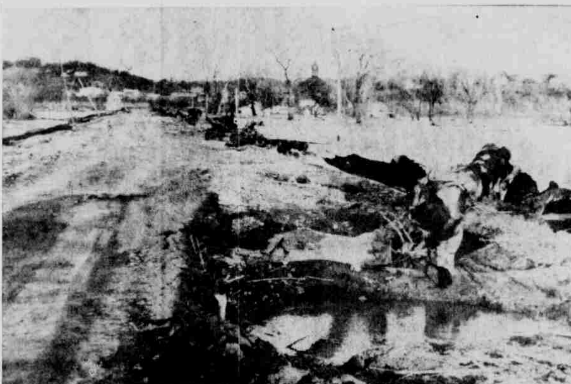
ROAD BATTERED—The county road east to the river here took a beating during the flood, being under 6 to 8 feet of water for 10 days. When the water went down last weekend, debris was left on the road and damage in the form of gaping holes in the grade showed up. The Army Engineers and Lloyd Morehead bulldozed the worst of the accumulation of logs and mud off the road to permit the Engineers to move to their headquarters on the Missouri River front Monday.
