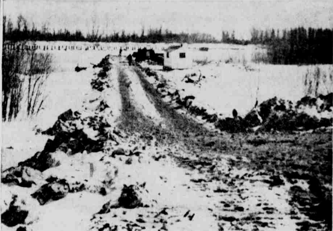
READY FOR WATER —The Army Corps of Engineers, in spite of snow and cold, went right ahead with the work of controlling the channel of the Missouri River here. Above is a dike which was under construction amid bad weather. Dikes are made of "rip-rap," quarry-run rock, for this one hauled about two miles from the Hebbner quarry south of Plattsmouth along the river.
