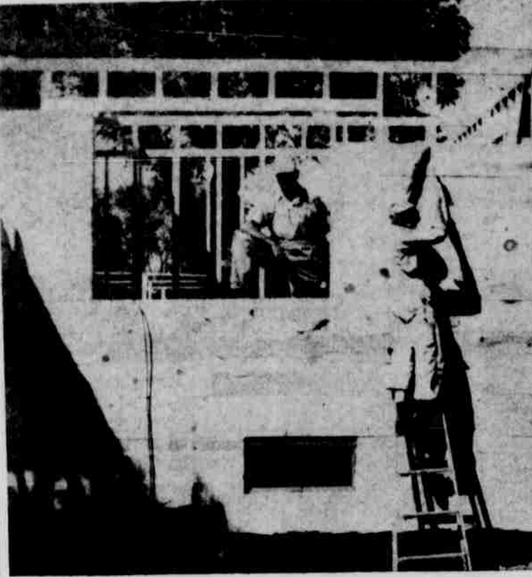
HERB CAMPBELL and Vern Hennings are just starting a remodeling job on the Chas Wondra home in Northwest Plattsmouth. The old part of the house, not shown in the picture is a two story affair with a spiral staircase which will be kept in the structure.
