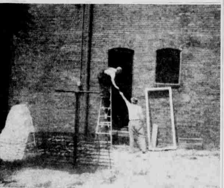
NO JAIL BREAK — There was an opening in the east side of County Jail here earlier this week but not much excitement about it. It wasn't a jail break. A door was being installed where a window had been for use as fire escape or delivering unruly prisoners to the jail. Sheriff Tom Solomon said that previously there was only one fire escape route. Working on the installation were contractor Carl Tiekotter, Plattsmouth, right, and LeRoy McCulloch Murray.
