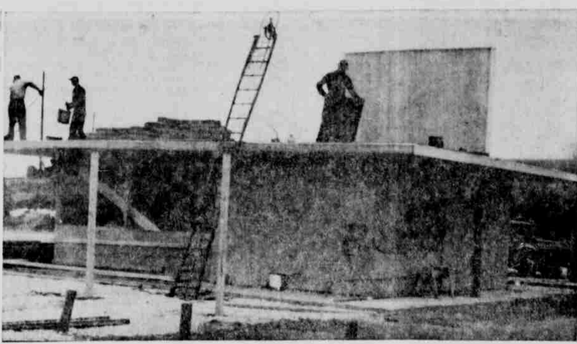
NEW BUSINESS AT LOUISVILLE — Workmen were putting a roof on this second unit of Jane's Drive-In when this picture was taken. Situated at Louisville just a short distance off Highway 50, it will feature refreshments for those who enjoy eating in their automobile. — Adv.
