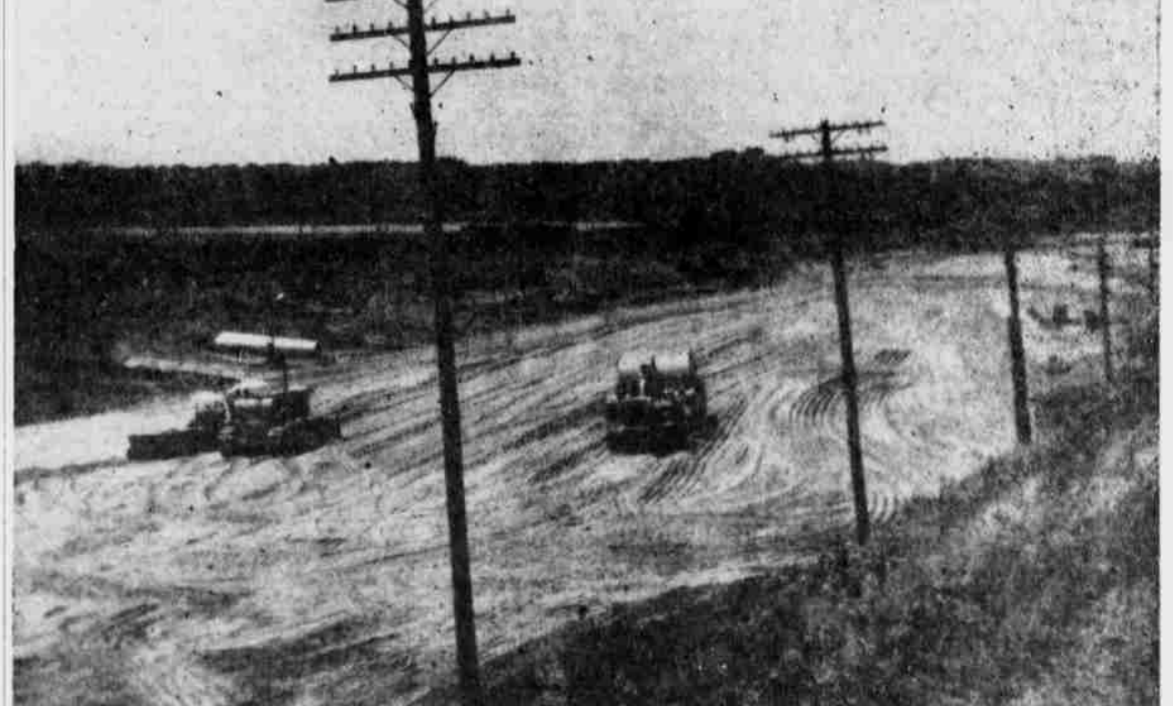
MANY TONS of sand have been moved into place by heavy equipment to provide a solid base for the new highway between Offutt Air Base and Plattsmouth. Work on the project has been going on day and night. This picture was taken near the Orespolis viaduct. (Journal Photo)
