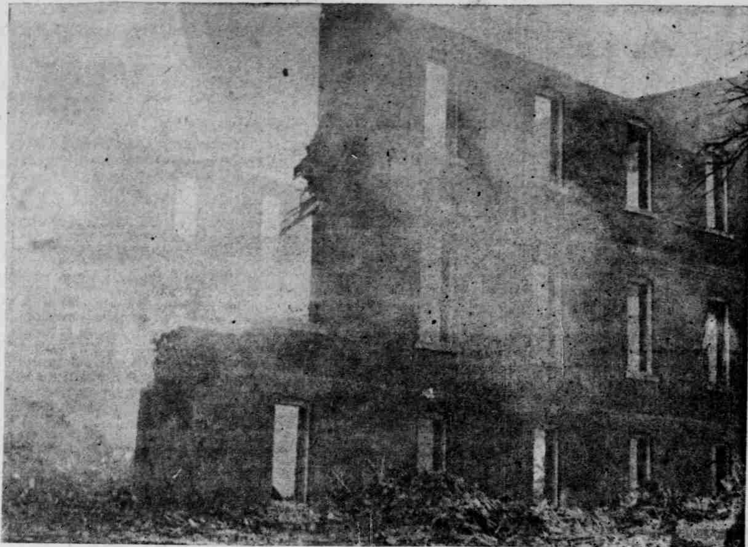
FIRE WAS one way to get rid of the rubble which collected inside the bare walls of this building being torn down at the Nebraska Masonic Home at Plattsmouth. Razers have now removed the insides of the three buildings which long served the home, and all that remained standing last week were part of the walls and lots of rubble.—Journal Photo.
