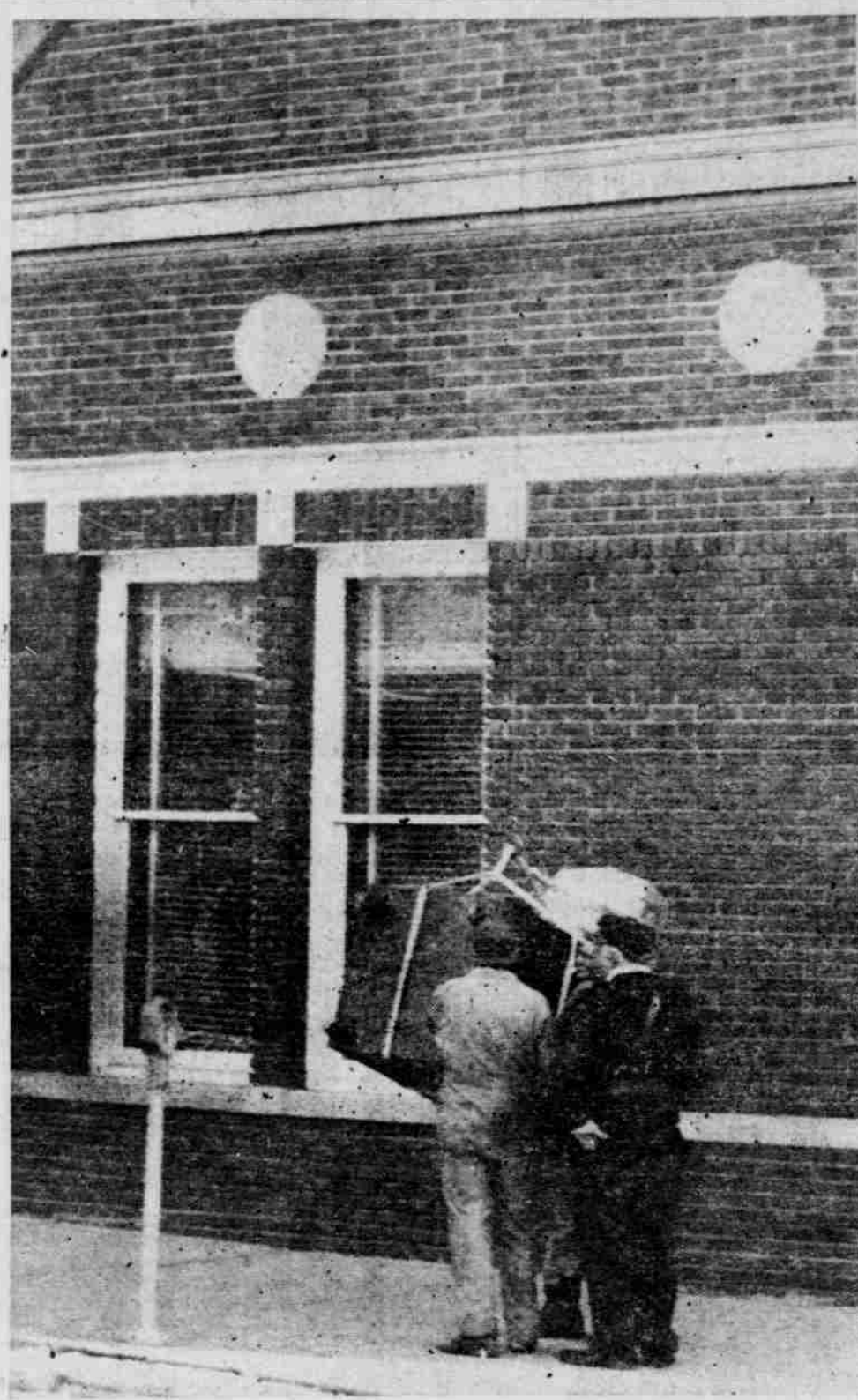
WAS CHIEF OF POLICE John Hobscheidt telling these two workers they would have to put a nickle in the parking meter, left, before they could stop holding up that safe and park it? It's doubtful and a crane is holding up the safe. This was a scene that attracted a large group of sidewalk superintendents at Plattsmouth Monday as Steve Davis moved a money safe out of his office.—Journal Photo.
