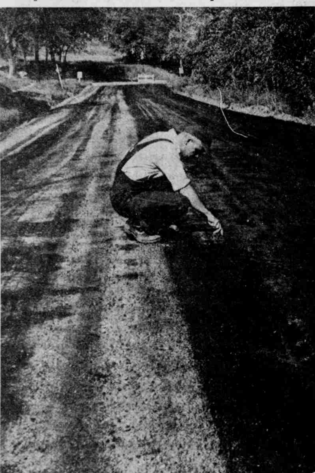
Councilman William Highfield, Platts-mouth street commissioner, is shown here checking the penetration of asphaltic oil poured on Lincoln avenue. The Northern Iowa Asphalt company put a penetrating coat on the dirt part of Shop avenue all the way to the Consumers Public Power District Substation this week. Left side of this picture shows road after sand coat was applied. This is the first treatment of three over a three year period which will be applied to this and many other blocks of Platts-mouth streets. The oiling is low-cost and is said to be durable.—Journal Photo.
