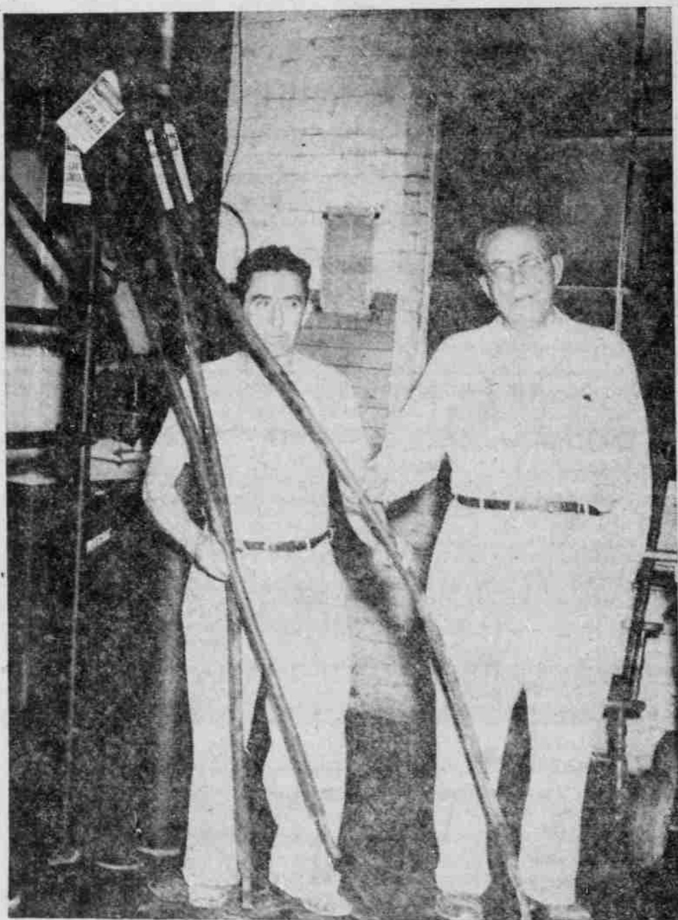
Beverly Sutton (a passerby) and Tom Hamlin, Plattsmouth Head of Consumers appliance department hold a part of a three-phase cable that failed plunging five county towns in darkness Monday night. Every male member of the local Consumers office was on the job in a matter of minutes restoring service as rapidly as possible.
