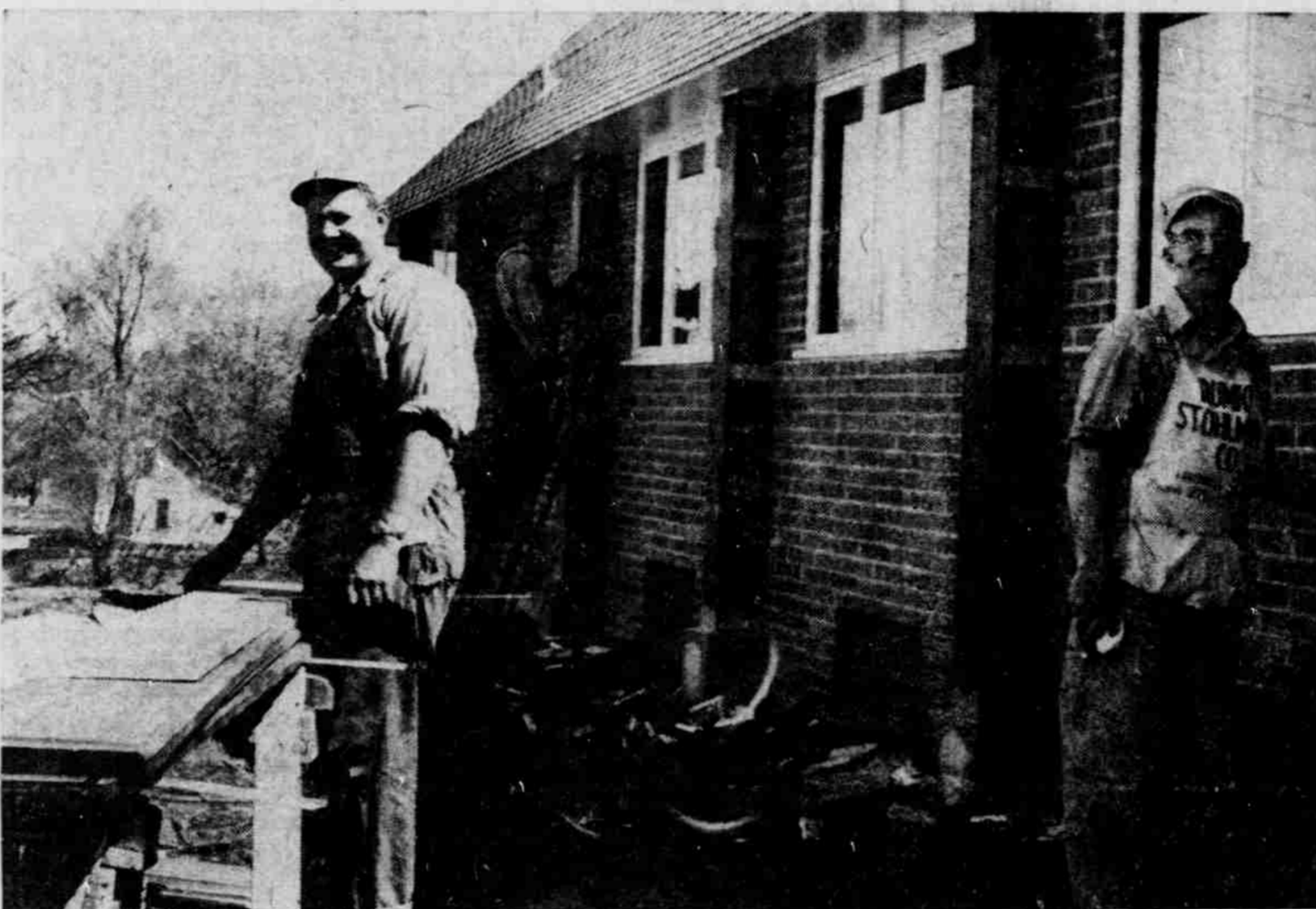
Hurrying to finish the new St. Paul's Lutheran church at Weeping Water in time for the dedication next Sunday are L. A. Baker of Weeping Water, left, nephew of Byron Baker, the contractor, Glen Taylor, right, and Verne Ackley, in the background of the ladder. Rev. Melvin Meyer is the pastor of the church congregation which has been using a temporary meeting place waiting for the finish of the new structure.—Journal Photo.
